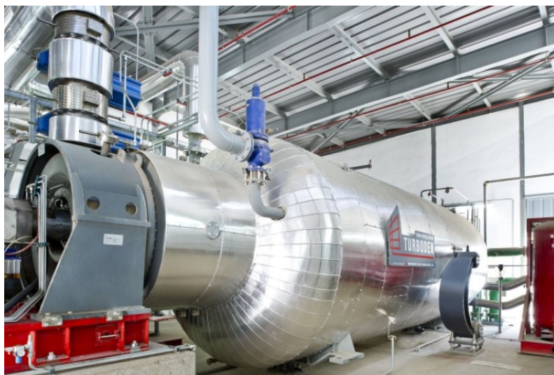
Geothermal Power ORC equipment identified
